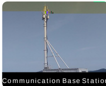
Communication Base Station
